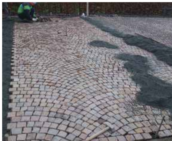
Figure 20.2 Private driveway using natural stone as permeable paving (courtesy The Ethical Stone Company/SteinTec)
