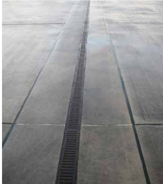
Figure 20.9 Macro pervious pavement in warehouse yard in north-west England with channel collection/pollution trap and concrete pavement construction (courtesy EPG Limited)
