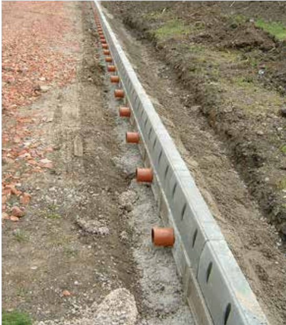
Figure 20.8 Macro pervious pavement under construction in the Midlands – kerb drain collector/pollution trap with connectors before placing diffusers and permeable sub-base to the left (courtesy Phil Tomlinson)
