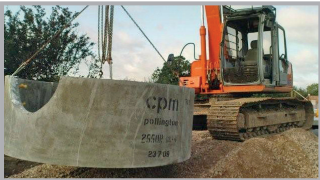
2550mm sectional installation, base chamber complete with half formed hole for 750mm pipe
