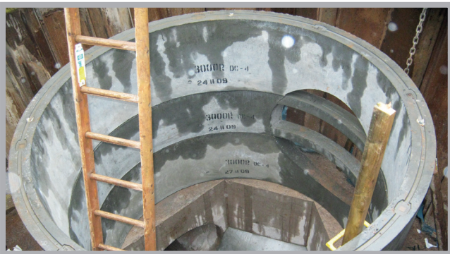
3000mm sectional chamber installation with a letter box opening for 1500mm concrete pipe
